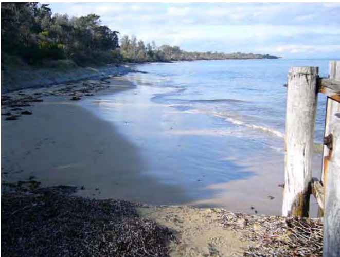
Erosion beyond eastern end of sea wall
